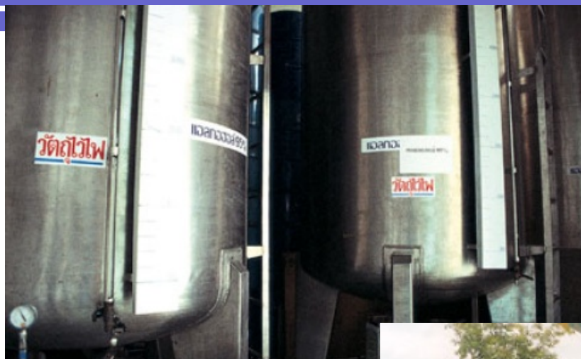
Alcohol storage tank
