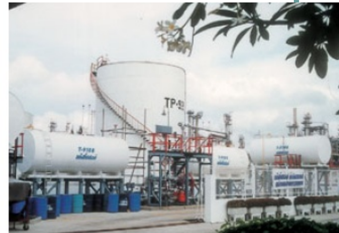
Gasohol blending facility at Bangchak Refinery
